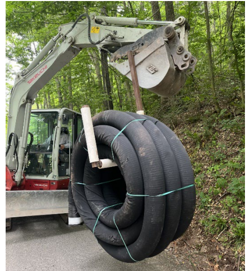
The Un-Reeler assists with the transport and installation of both 100 feet long reels of 6 inch diameter underdrain and 60 feet long reels of 8 inch diameter underdrain. Photo: Lewis Township, Lycoming County
