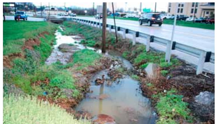
An enclosed surface water drainage facility under a township road in York County empties into a parallel open surface water drainage facility along a PennDOT highway. Trash and accumulated sediment lead to poor drainage in the upstream area. Photo by Michael H. Fleming, ISMF LLC.
