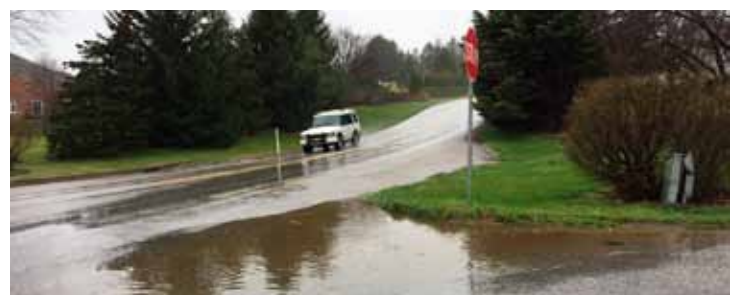
This open surface water drainage facility in York County is not functioning as designed due to paving overlay and inlet location. Photo by Michael H. Fleming, ISMF LLC.
