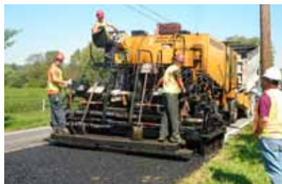
A single paving machine applies the polymer modified emulsified asphalt membrane overlaid with an ultra-thin bonded wearing course of hot-mix asphalt concrete in one pass. (PennDOT photo)
