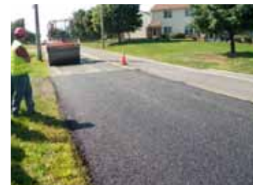
UTWC is placed in one lift with a final thickness of one to one and a half times the diameter of the coarsest or maximum-sized aggregate. (PennDOT photo)
