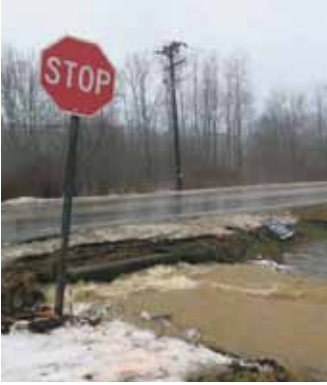
A subsurface water drainage facility in Warren County overflows after warm temperatures and heavy rainfall prove too great for the pipe under the road to handle. Photo by Stacey Gross, Times Observer.
