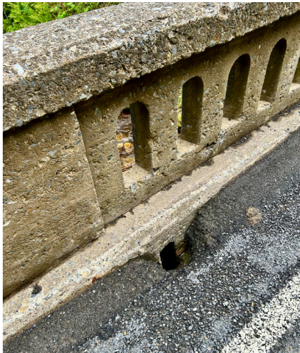
A simple older drop through scupper in a concrete barrier that has been cleaned and maintained. Photo: ISMF LLC
