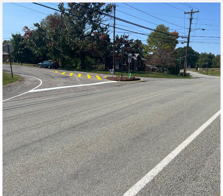
Figure 3: After installation of pavement markings and signage, improvements can be seen looking from SR 989. Photo: PennDOT LTAP
