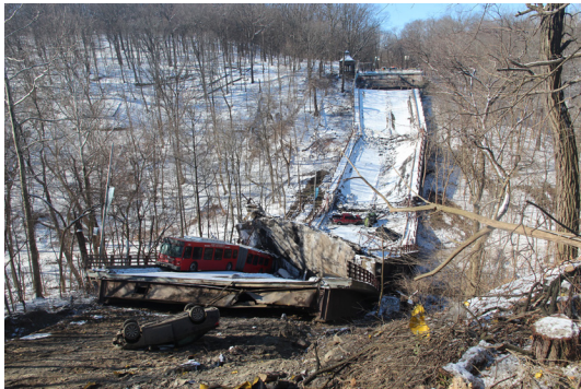
A west-looking view shows the collapsed Fern Hollow Bridge from January 2022. Photo: NTSB
