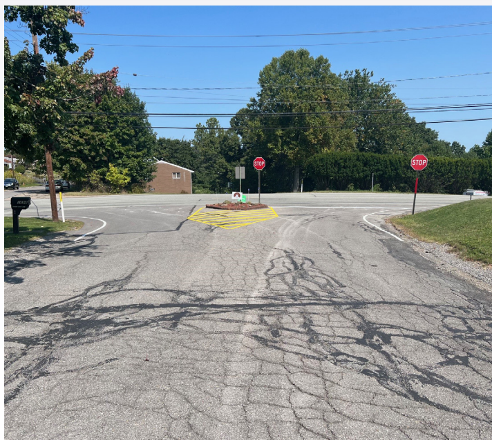
Figure 2: After installation of pavement markings and signage, improvements can be seen looking from Longvue Circle. Photo: PennDOT LTAP
