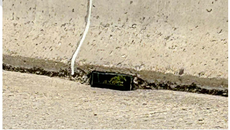
A simple drop through scupper seen here at the base of a concrete barrier that has been cleaned and maintained. Photo: ISMF LLC
