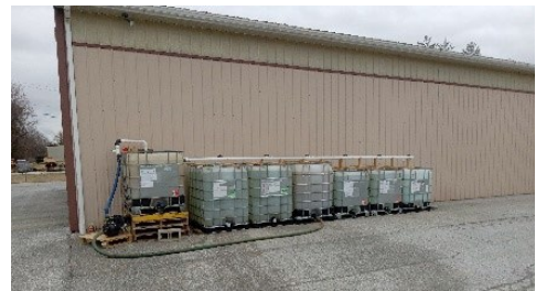
The photos are showing the brine maker the borough build and the totes that store the brine. Photo: McSherrystown Borough, Adams County
