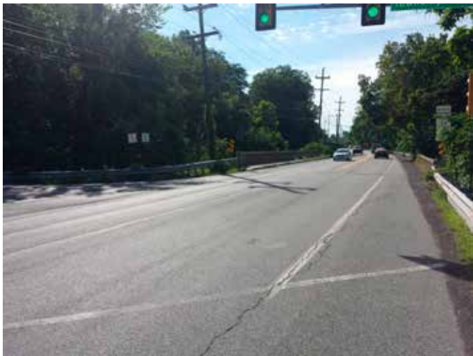
The bridge site near approach load posting sign (at right) is visually obstructed by vegetation growth.
