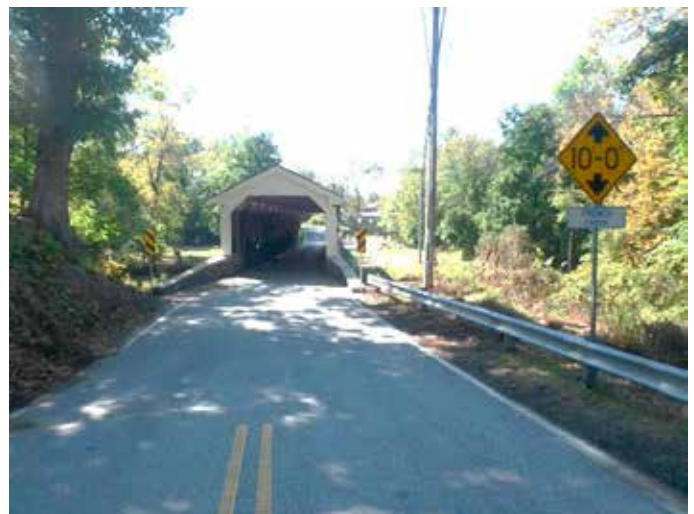
The bridge width here is substandard compared to the approaching roadway. Note the hazardous clearance markers at the bridge.
