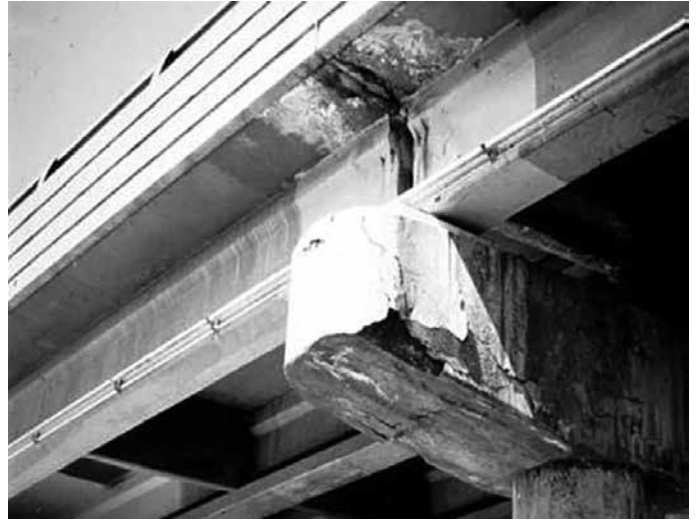
Leaking deck joint. Credit: FHWA
