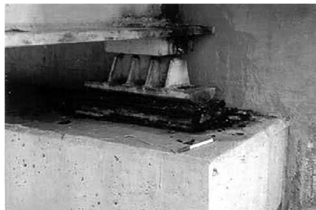
Deteriorated steel rocker bearing. Credit: Ohio Department of Transportation
