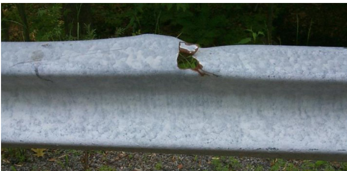
High-severity deterioration of the W-beam rail
