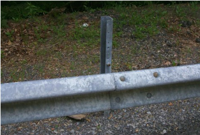
W-beam panel disconnected from the post
