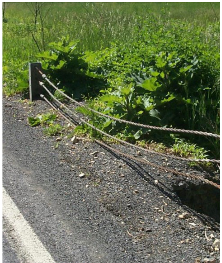
Medium-severity cable sag
