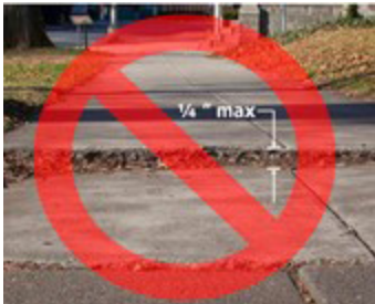
The elevation difference between two pieces of sidewalk may not be more than 1/4 inch.
