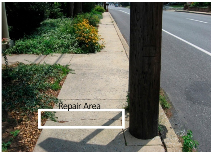
Minor repairs, such as filling in cracks, does not trigger ADA compliance.
