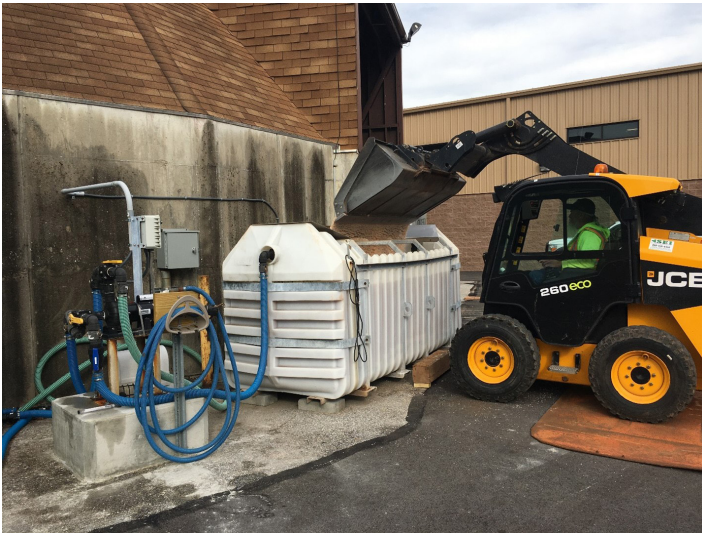
Dover Township, York County, produces its own salt brine by mixing sodium chloride (road salt) purchased through the Department of General Services with potable water to produce a 23.3% mixture.
