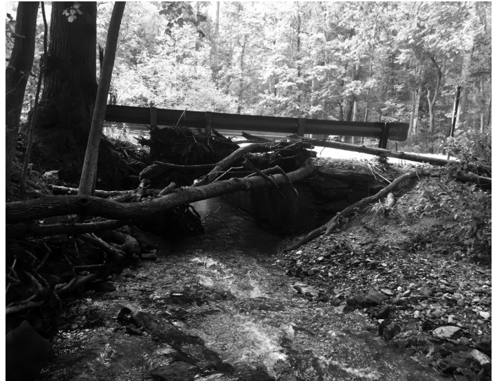
The steel beam bridge with a steel grate deck survived the flood, but debris needed to be removed and the bridge was inspected for safety.
