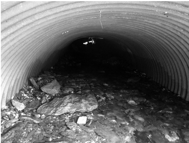
A flood event caused the municipal culvert to fill with debris. Include the cost estimates to remove debris in culverts.
