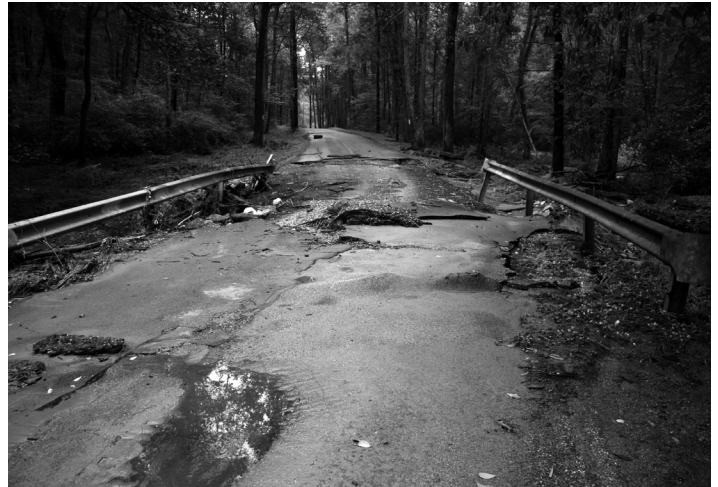
This is Line Road in North Hopewell Township. This was a localized event that did several million dollars of damage to township infrastructure. Take photos before any work is done to show the true damage.
