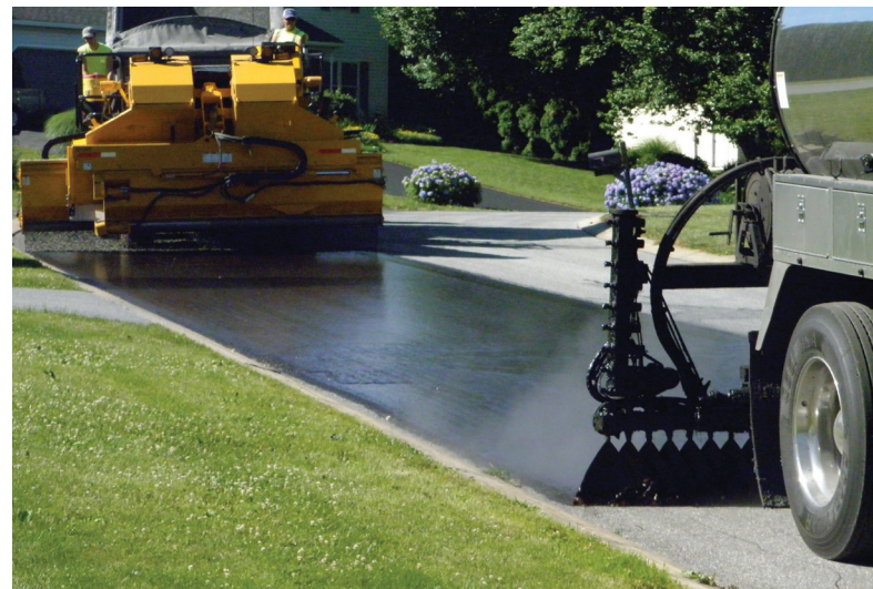
Emulsion is being applied as it is followed closely by a chip spreader as suggested in the specifications. Photo: PennDOT
