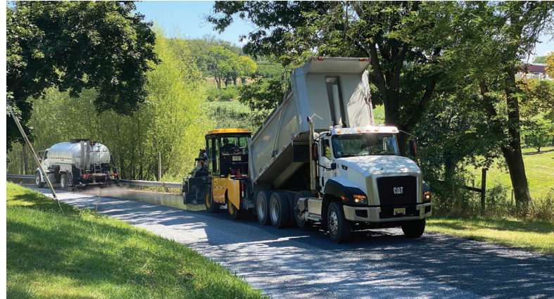
An emulsion distributor truck at work followed by a calibrated chip spreader and dump truck with #8 aggregate. Photo: PAAMA
