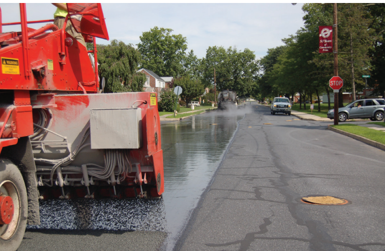
A calibrated chip spreader at work along a residential street distributing #8 aggregate. Note that manhole covers are protected so that emulsion and aggregate do not adhere to the cover. Photo: PAAMA
