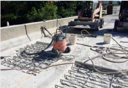
Contractors working within a municipality should follow the MS4 requirements even on a county- or state-owned bridge.
