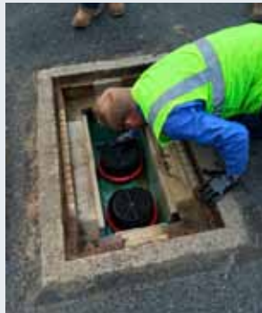
Stormwater inlet with filtering devices to trap fine sediment.
