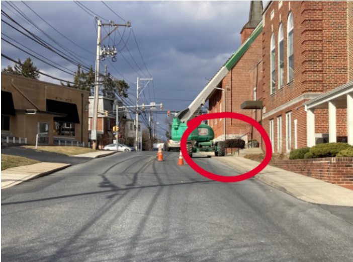
Figure 11: A work area that blocks a sidewalk, and forces pedestrians into conflict with traffic.
