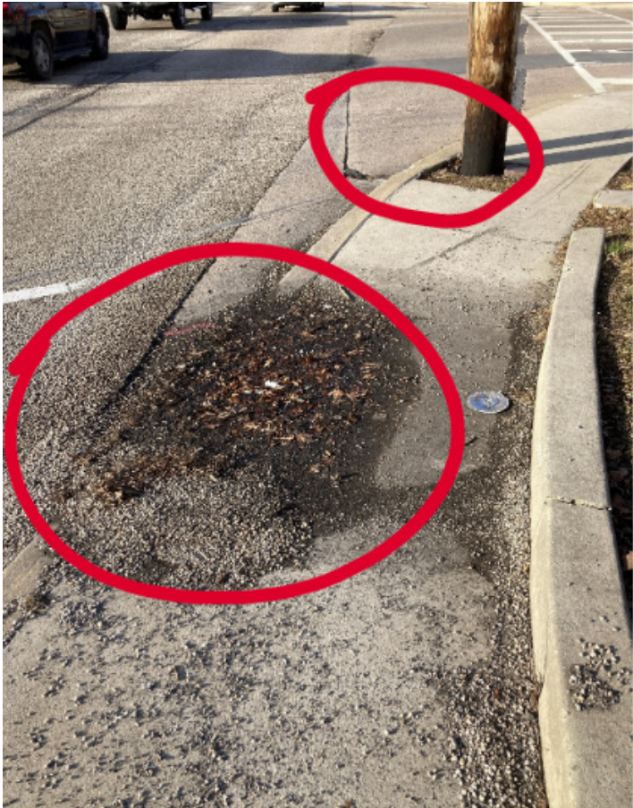
Figure 9: Ponding and other drainage issues can limit the functionality of a sidewalk and/or ramp. Also note the utility pole restricting the width of the sidewalk and PAR.
