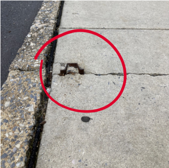
Figure 10: Old signposts and other objects can be tripping hazards and not compliant with the ADA. ADA identifies any protruding object over ¼ inch as a hazard.
