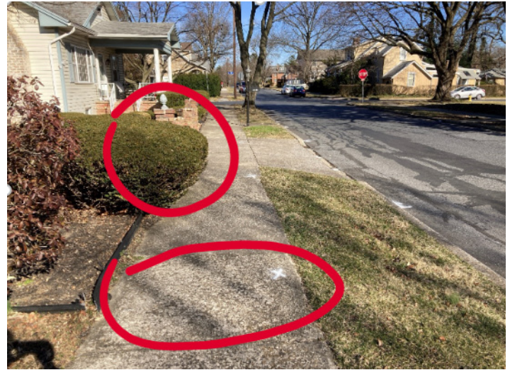
Figure 4: This photo shows vegetation limiting the width of the sidewalk, and a sidewalk panel that is not smooth and in need of repair or replacement.
