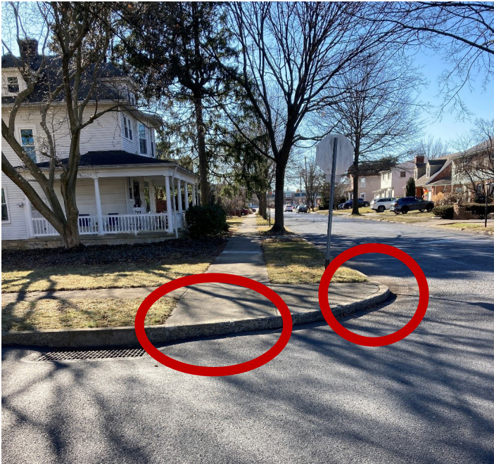
Figure 6: No curb ramps are present here.
