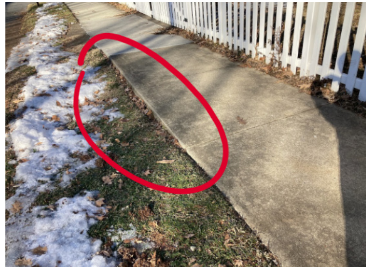
Figure 5: Edge drop-offs can be tripping hazards.
