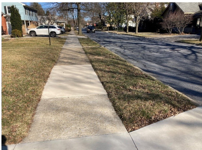
Figure 3: Per ADA and PennDOT standards, sidewalks shall be smooth, stable, and slip resistant. This shows a repaired section of sidewalk.
