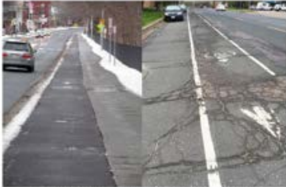
Figure 15-1: Examples of Debris, Faded Markings, and Snow Clearing
