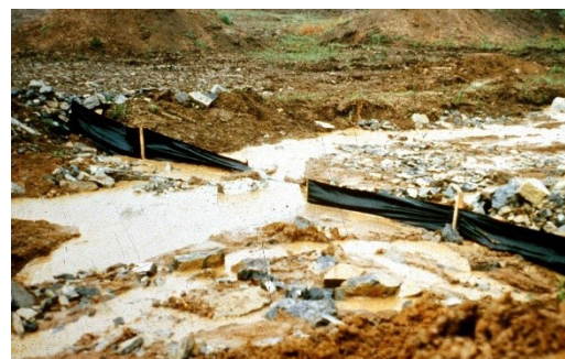
A silt fence fails after being placed across an area of concentrated flow.
