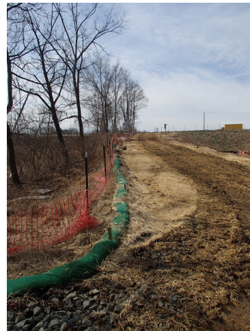
A compost filter sock is improperly placed downhill along an access road.
