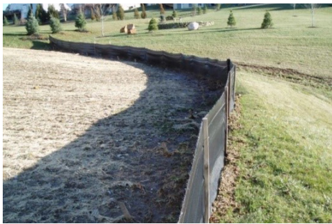
Silt fence properly placed at an even elevation (York County Conservation District)
