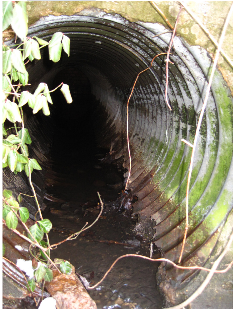
Pipe deterioration requires retrofit repairs. Photo: NTM Engineering, Inc.
