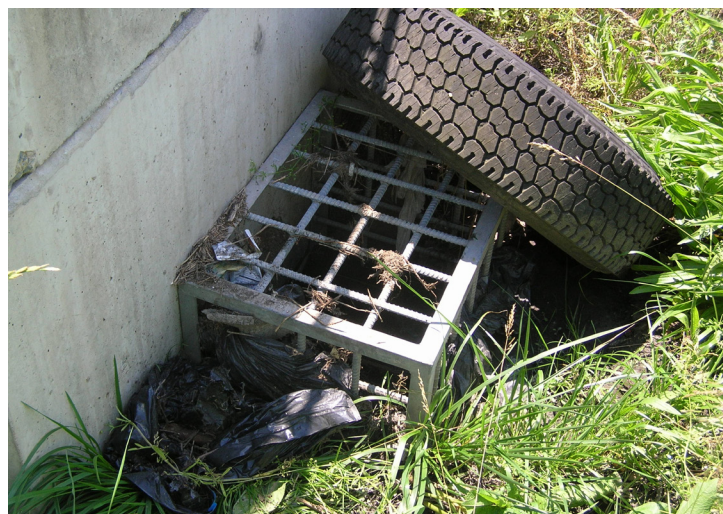
Trash and debris accumulation at a basin outlet structure should be removed and cleaned up. Photo: NTM Engineering, Inc.
