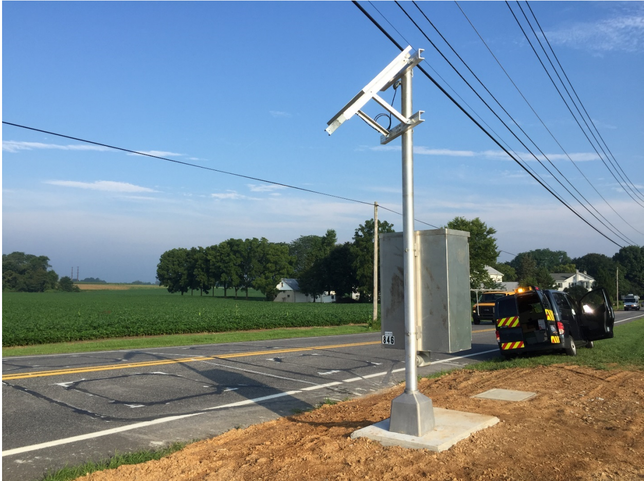
CAVC 846 in Cumberland County
