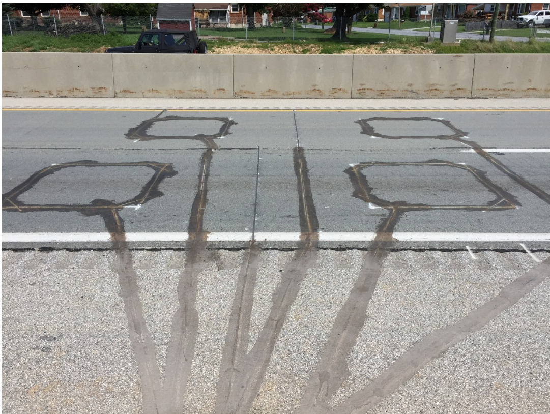
CAVC 205 Sensor Array on I-83 in York County
