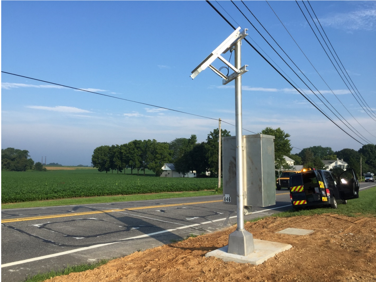
CAVC 846 in Cumberland County
