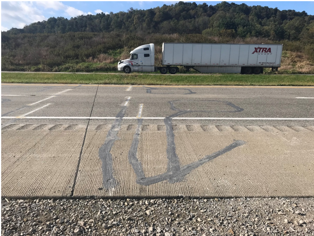
WIM 706 Sensor Array on I-79 in Greene County
