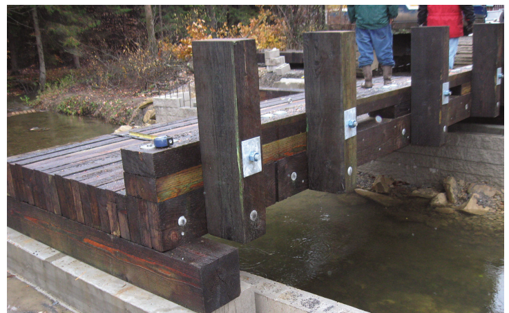
DURING: With the help of neighboring municipalities and local contractors, Huston Township used its own equipment and workforce to employ the Geosynthetic Reinforced Soil-Integrated Bridge System alternative technology.
