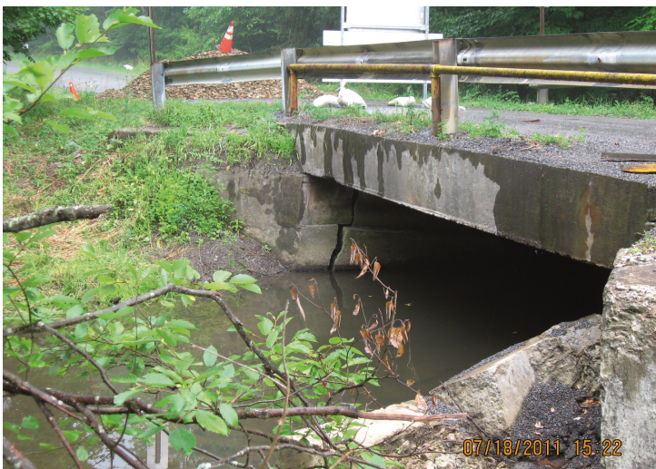
BEFORE: The bridge had deteriorated to the point that it was unsafe for vehicles to cross it.
