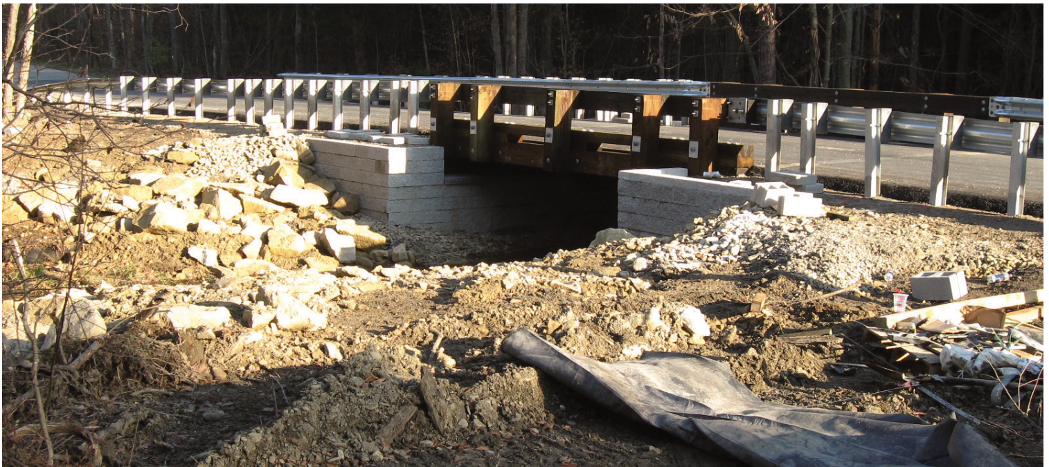
AFTER: After 35 days of work for the price of $102,000, Huston Township was able to reopen the bridge in record time.
