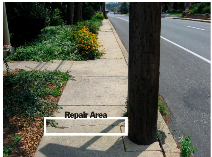
Minor repairs, such as filling in cracks in a sidewalk, do not trigger ADA compliance.
