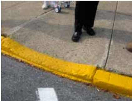
Old ramps can be barriers to access.
