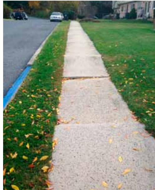
Poorly maintained sidewalks can create barriers to access and can be safety hazards.
