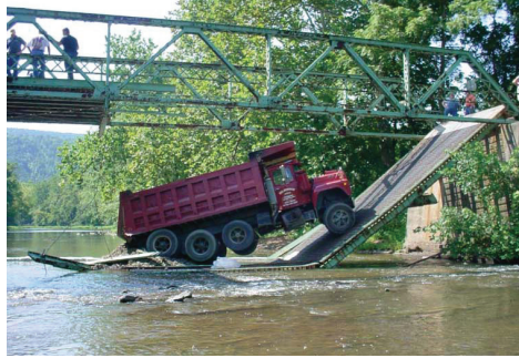
A truck fails to follow the 15-ton weight restriction posted on a truss bridge over Shermans Creek.
