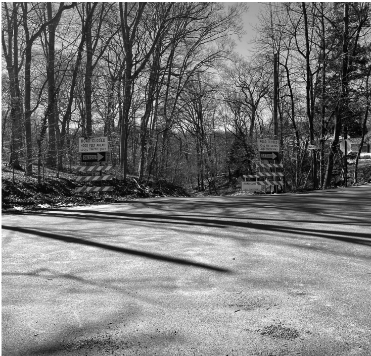
Figure 3 shows where the road closure was and the detour onto S. Ridley Creek Road.
