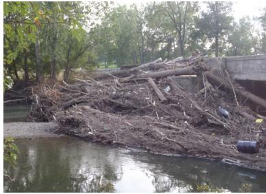
Debris damming by a bridge after the fall 2011 flood. (Photo courtesy of PennDOT)
