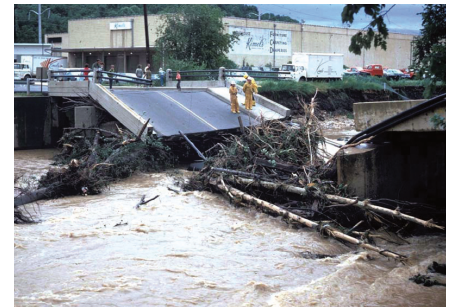
Bridge failure from debris damming. (FHWA-IF-04-16, Hydraulic Engineering Circular No. 9)
