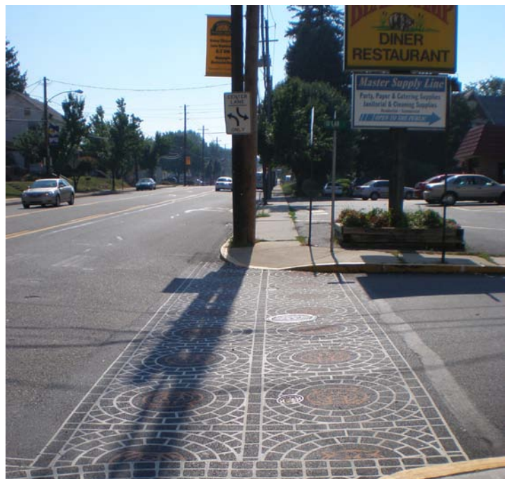
Example from Macungie, Pa. This pattern/style does not meet current standards and also lacks the transverse white reflective lines.
