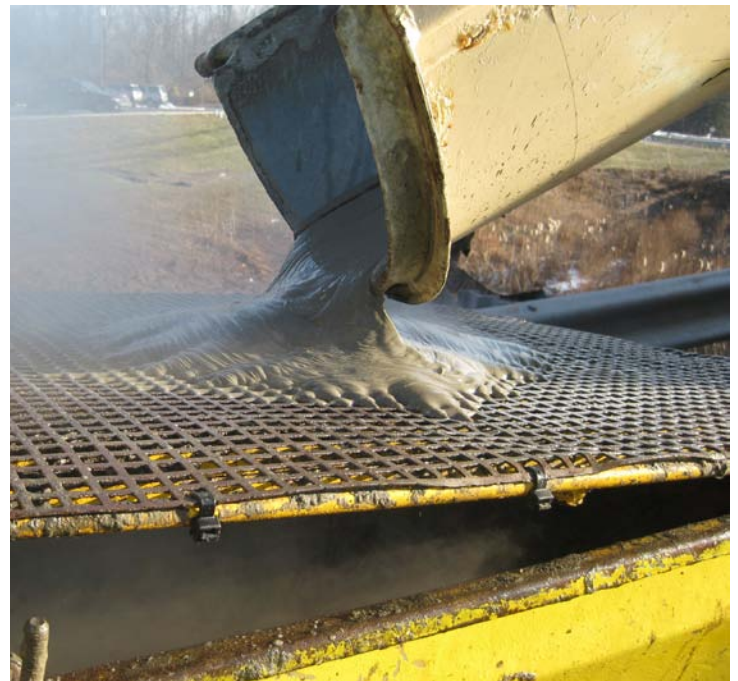
and then “pea soup” gravel is pumped into the space between the new liner and the old pipe. Here, the grout is being dumped from the concrete mixer into the concrete pump.
