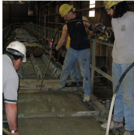
Immersion vibrators are used for consolidation of the concrete. In some cases, hand methods such as rodding or spading are sufficient.
