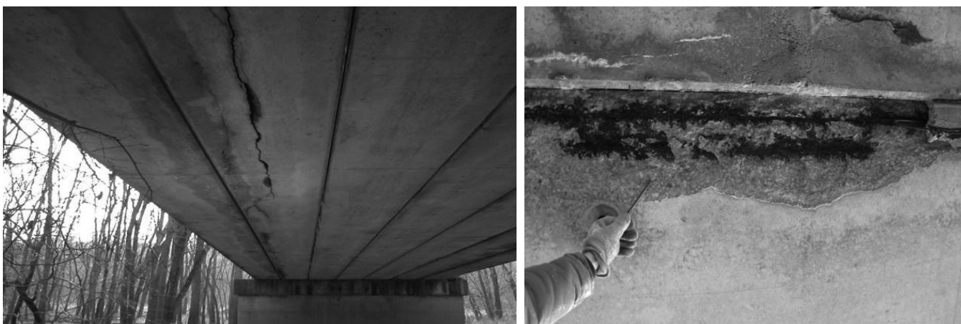
Figure 4: Longitudinal cracking (left) and spalling and delamination (right) induced by corrosion of the steel reinforcement
