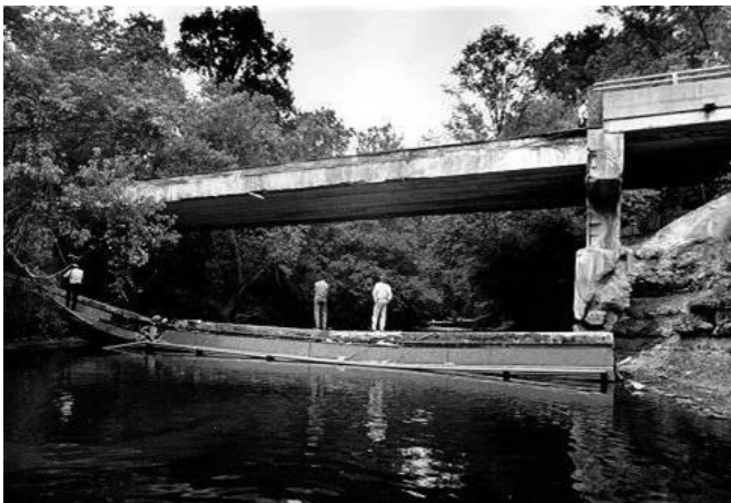
Figure 5: Prestressed bridge beam failures in Pennsylvania and Ohio
