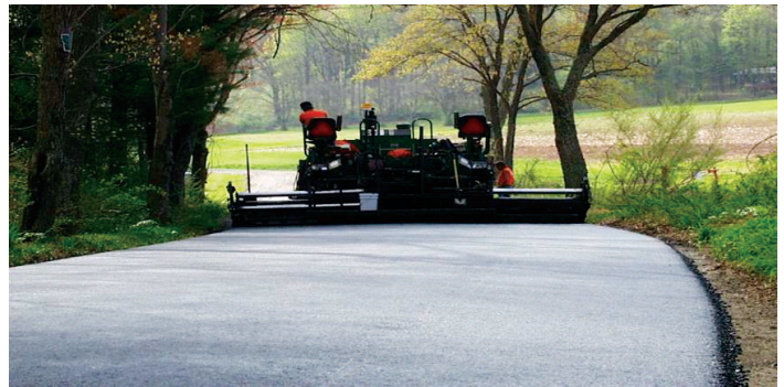
Palestine Road in Wayne Township, Schuylkill County, receives final paving. Since 3 inches of 19-mm SUPERPAVE were placed over top of the FDR at this location in 2009, the road has not needed any maintenance.
