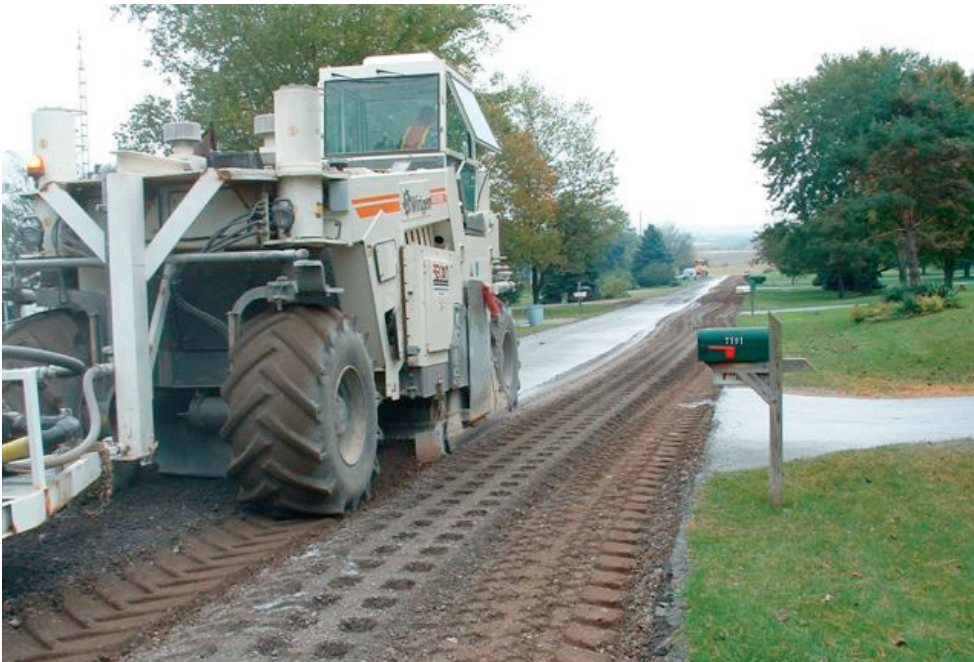
Lime/fly ash is mixed after the pulverization pass is completed on this FDR project near the Mason-Dixon Line.
