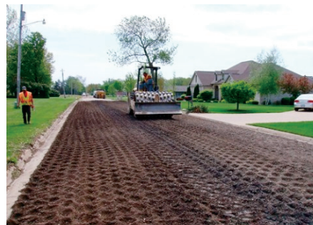
(left) During bituminous stabilization FDR, such as on this road in Robesonia borough, the breakdown compaction takes place immediately after the emulsion break and can be followed with motor grader shaping. (right) A vibratory pad-foot roller compacts the FDR mixture.
